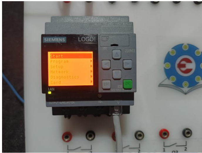
Gambar 1 : Uji Coba Transfer Data Ke PLC Siemens LOGO!
